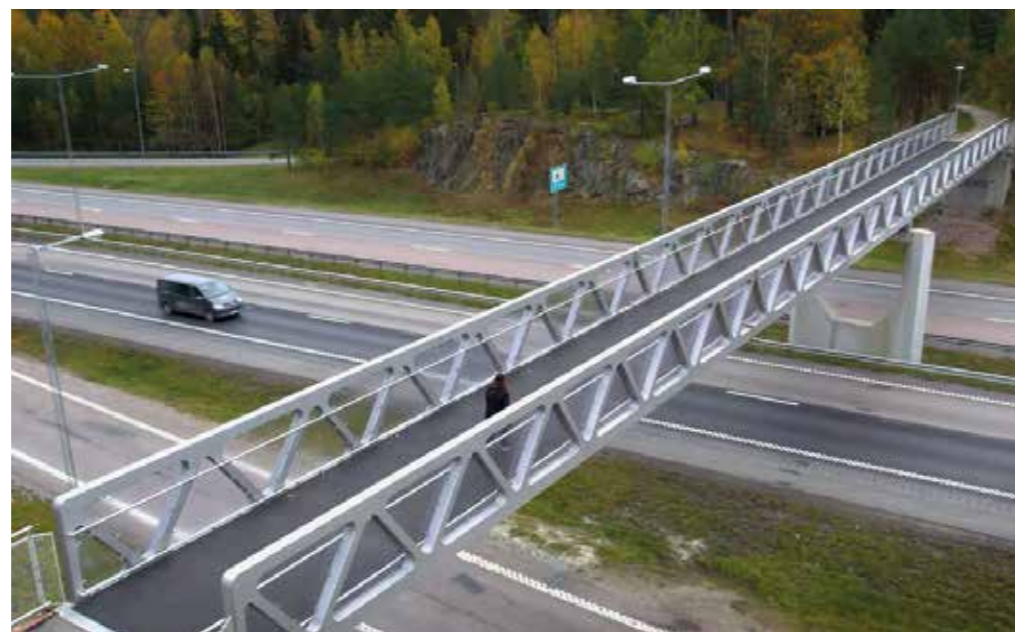
The Södertälje bridge contains several different grades of duplex, with standard austenitic grades used for some non-structural components.
