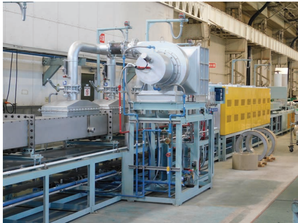
New BA furnace installed
