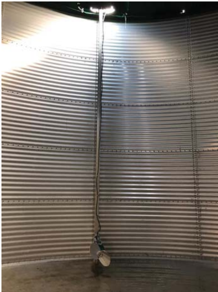
Stainless steel mixer inside slurry tank made of stainless steel
