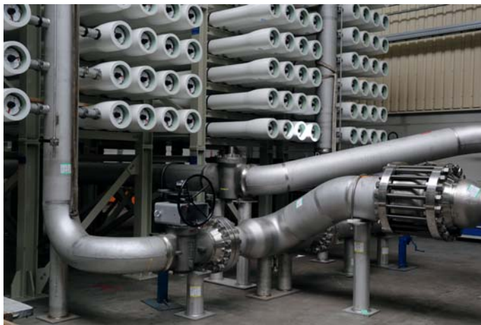
Skids for seawater desalination in superduplex.
