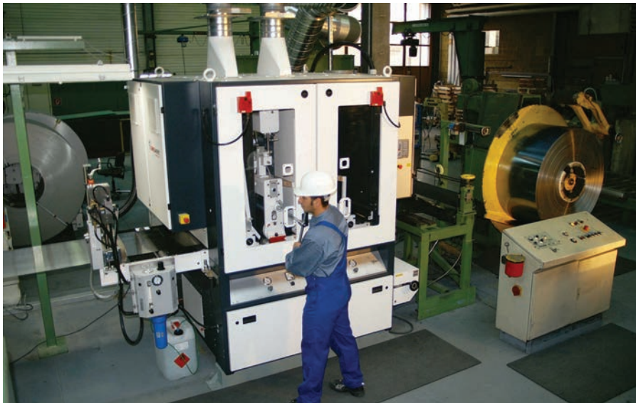
Another close up of machinery installed at Vogel-Bauer Edelstahl.
