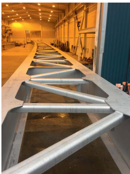
The use of prefabricated modular duplex components allowed the Söderströmbron bridge in central Stockholm to remain open to traffic during repairs, minimizing traffic disruption.
