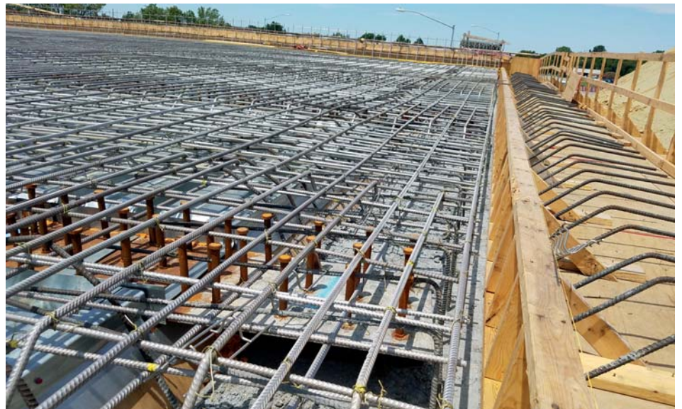
The intermodal connector project in Norfolk, Virginia is utilizing over 500 metric tons of Forta DX 2304 duplex stainless steel concrete reinforcement for highway bridges in the coastal area near the Port Of Virginia.
