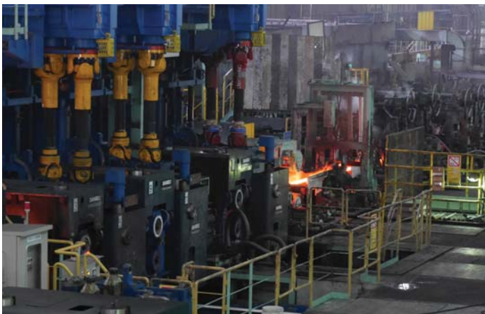
The company completed the replacement of its bars and wire rods rough rolling mill this year.
