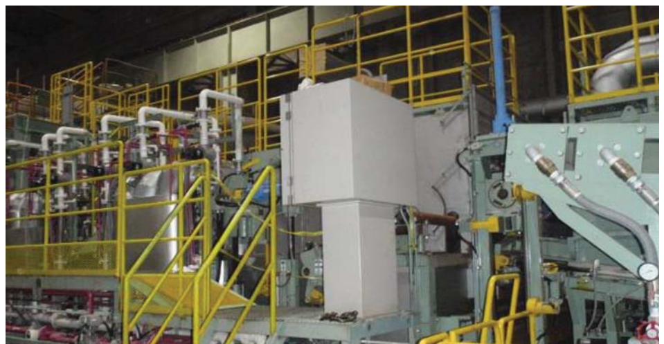
The annealing-pickling line for cold rolled products was recently remodelled.
