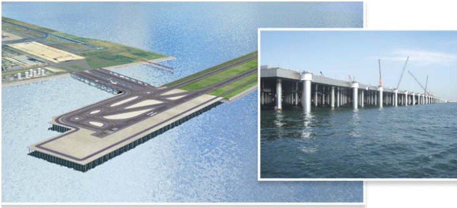
270 is adopted as the lining jacket for the pier construction of the new runway at Haneda Airport, based on its high corrosion resistance which is comparable with titanium.
