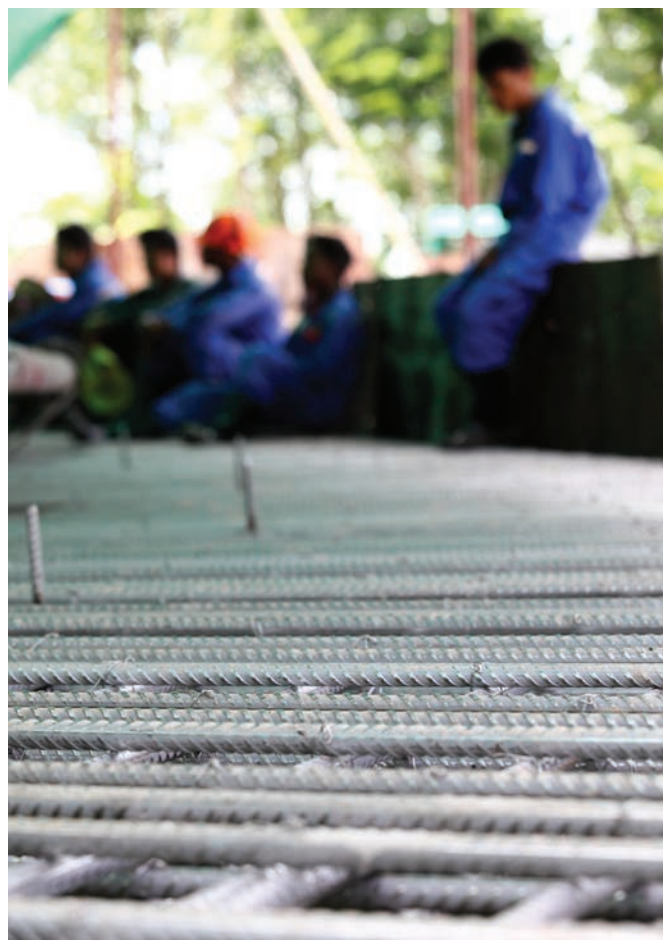
Talk about sustainable: this Buddhist temple in Thailand is designed to last over a thousand years. Outokumpu duplex LDX 2101 ® reinforcement bar (rebar) was used in the most critical concrete structures. Photo courtesy of Surachet Amnuaywittayakul
