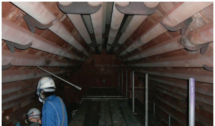
347AP furnace tubes in hydro-cracker
