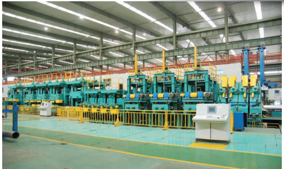
The new 24" continuous welding line for the production of high-quality pipes with a long length without circumferential welding.
