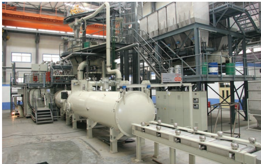
Electron beam cold hearth melting furnace (EB furnace)
