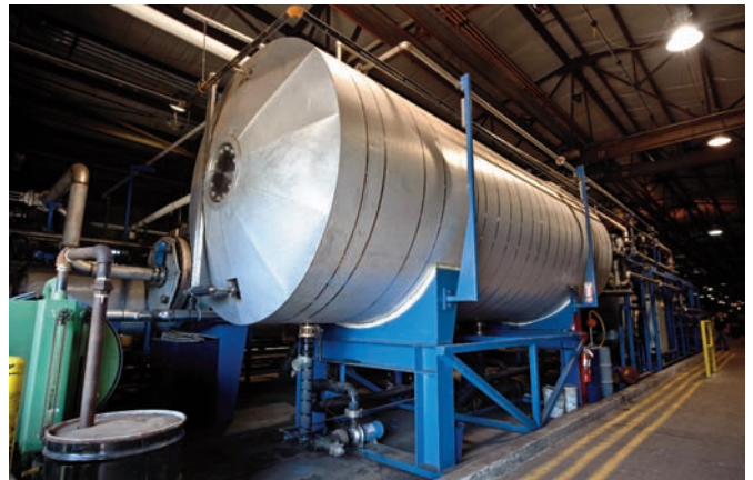
The environmentally-gentle degreaser in RathGibson – Clarksville.
