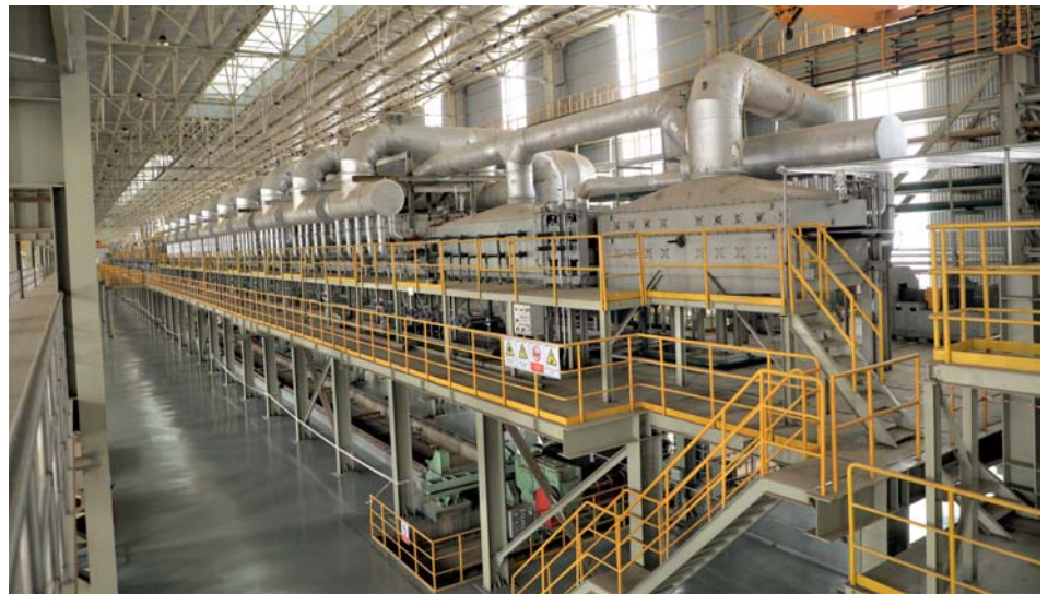
Chromeni Steel’s continuous inline annealing furnace.
